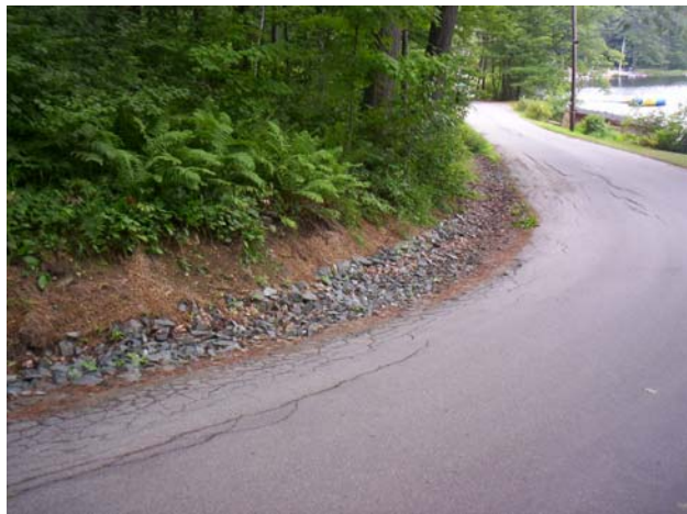
Rip rap swale along road to dissipate stormwater volume, reduce erosion and stop harmful pollutants and nutrients from entering the surface water.
