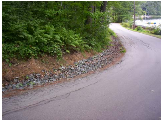
Rip rap swale along road to dissipate stormwater volume, reduce erosion and stop harmful pollutants and nutrients from entering the surface water.
