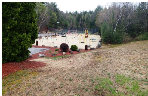
Eroding slope. Date: 5/2/17
