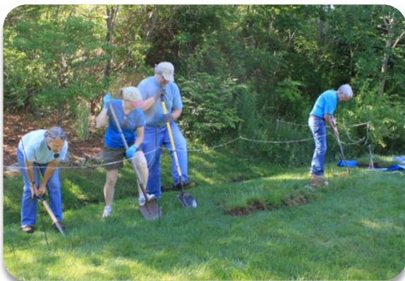
The SOAK crew removing sod in the rain garden area. The channel that the rain garden will intercept is visible behind the crew.
