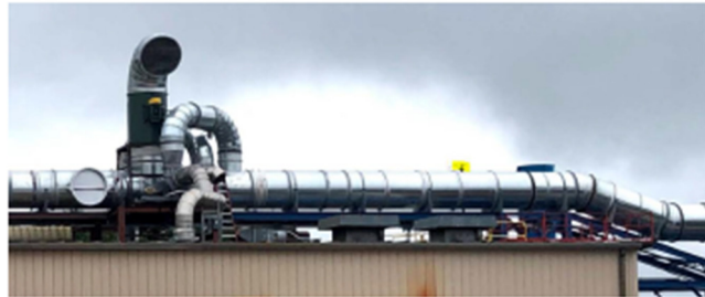
FIGURE 2 TEST PORT LOCATIONS RTO INLET DUCT
